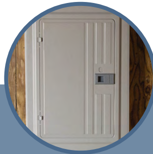
150AMP SUB-FEED LOAD CENTER FOR CO-LOCATION AREA
