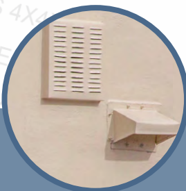
LOUVERED INTAKE AND ELECTRICAL PENETRATION
